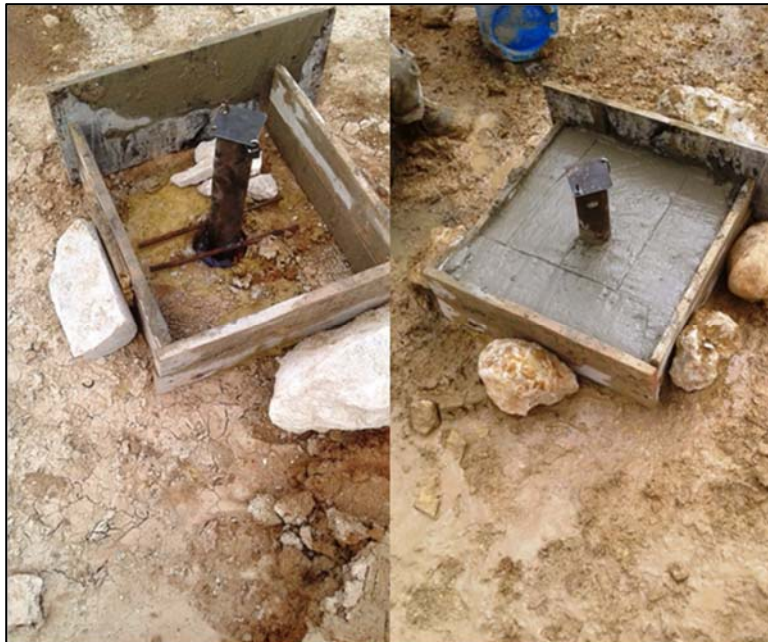
Figure 8 Open standpipe piezometer.
